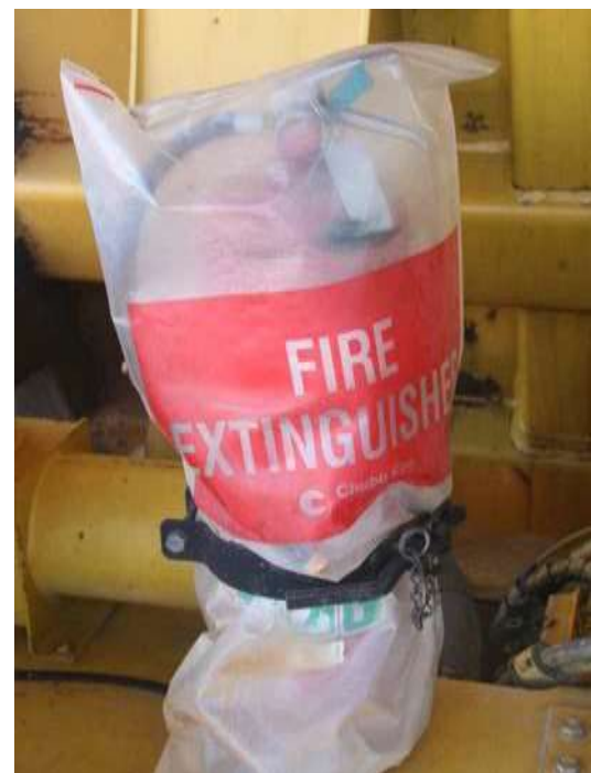
Handheld Fire Extinguisher
