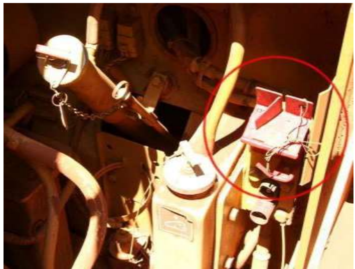
Battery Isolation Switch
