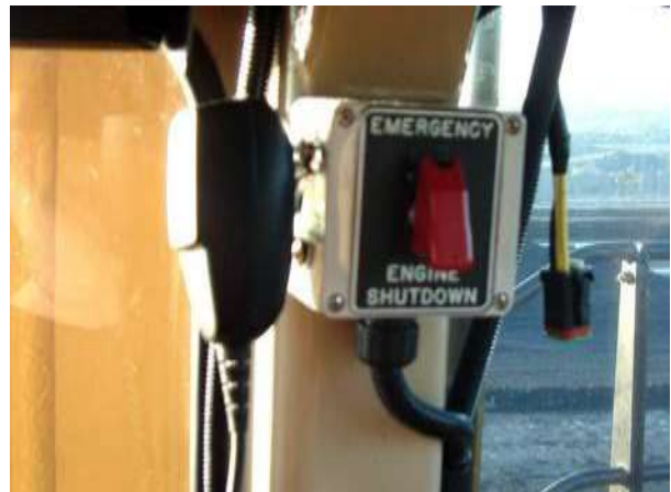
Cabin Emergency Stop Switch
