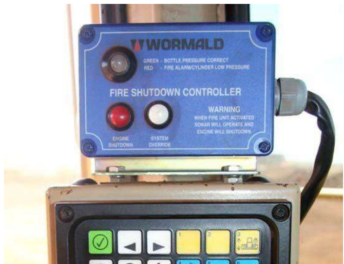
Fire Shutdown Controller
