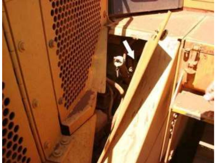
Battery Isolation Location
